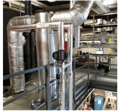
The buildings are heated via a central heat generation and distribution system fired by biomass from the local area: specifically, a pellet-based system producing 350 kW with 22 kW of waste heat recovery. This generates an extra 63 MWh of energy a year, enough to heat ten homes. The pellet system provides up to 92% of the heat required. The waste heat produced in cooling the offices and ventilating 22 housing units is also utilised. An efficient gas condensing boiler with an output of 400 kW is on hand to cover peaks in demand. Photo: SIR
